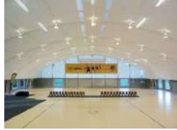
Tensioned ceiling - Sports hall (NZ)
