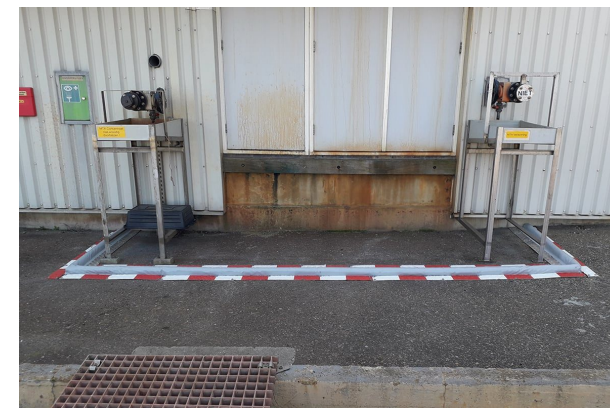
U-shape around a filling point, with red-and-white warning marking
