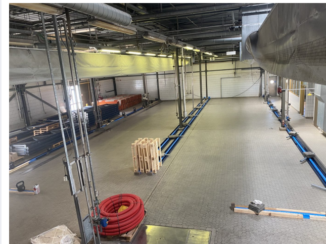
Sills installed in a production hall with forklift traffic
